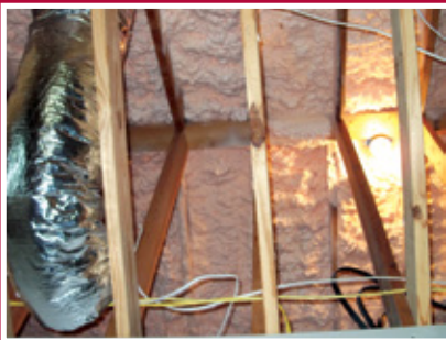
GacoFireStop sprayed in the attic around a heat duct and a light fixture.
